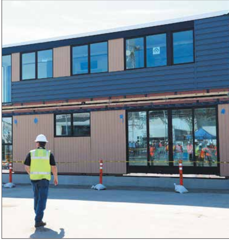
Southern California Gas Co. has kicked off the assembly of its H2 Hydrogen Home in Downey, the first of its kind in the United States that will show how carbon-free gas made from renewable electricity can be used to fuel clean energy systems of the future. (Photos by Alex Dominguez)
