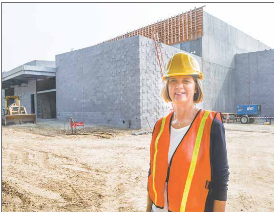
Principal Lisa Reed stands in front of the gym at La Mirada High School where they are in the first phase construction. (Photo by Keith Durlfingler)
