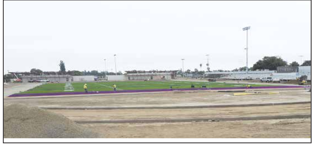
The stadium at Norwalk High School is gaining progress with the hopes of the football team to use it when it is completed in December. (Photo by Keith Durlinger)
