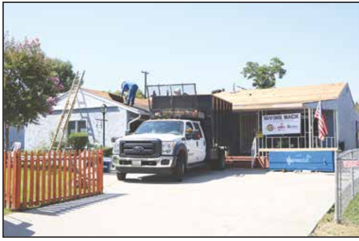
The new roof was entirely donated through the efforts of Owens Corning and Habitat for Humanity. (Photo by Alex Dominguez)
